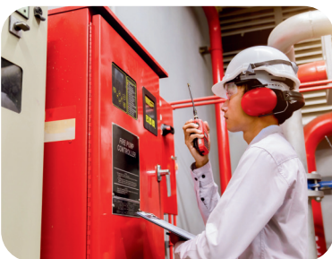
Fire Safety Service
